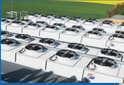
▲ AGVH-type Güntner FLAT Vario condensers each with 595 kW/2,030 MBTU/h have been designed as special units due to building regulation noise specifications of 50 dB(A)/10 m (33 ft) in order to achieve the specified operating parameters.
